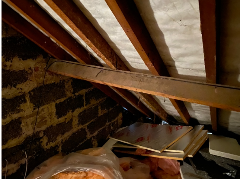
Photograph 5: Within the loft void showing gaps within the soffit as daylight shines through.
