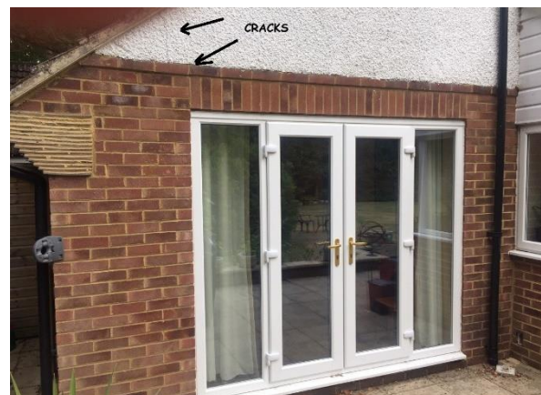
Cracking to the rear elevation of the right-hand extension
