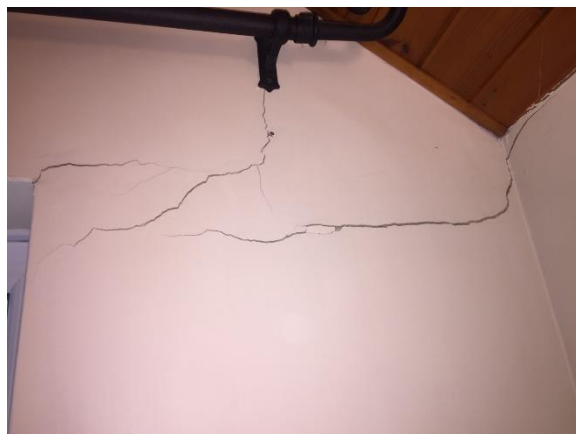
Diagonal cracking to the rear wall of the right-hand lounge
