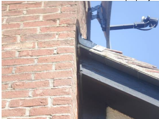
Photograph 10. Gap between timber and chimney stack at rear of the property
