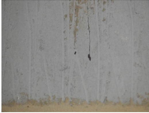
Photograph 17. Bat dropping on blockwork gable end wall
