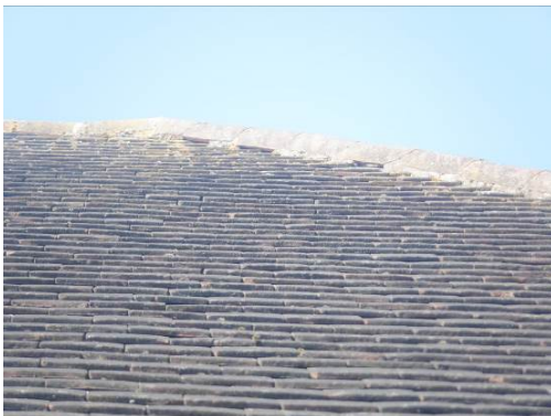
Photograph 5. Gaps in hip tiles on the eastern roof elevation
