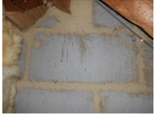
Photograph 16. Bat droppings on blockwork gable end wall
