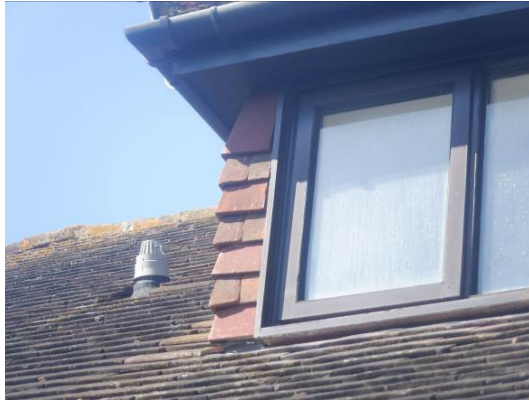
Photograph 8. Gaps in hanging tiles around corner of the dormer window to the east of the property
