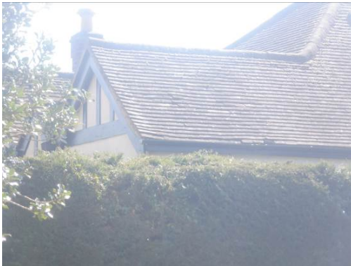
Photograph 3. Lifted plain roof tiles at the western side of the property
