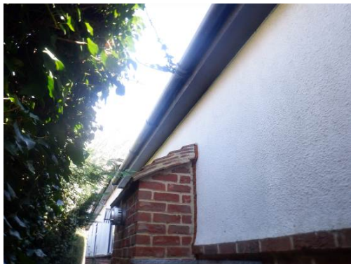
Photograph 11. Tight timber soffit boxes
