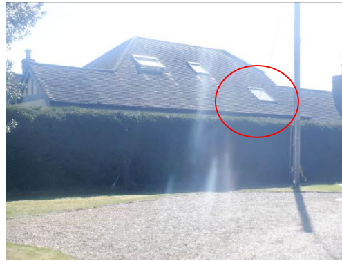
Photograph 4. Lifted plain roof tiles around window at western side of the property
