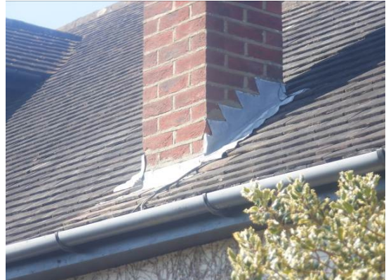
Photograph 9. Gaps in led flashing around chimney to the east of the property
