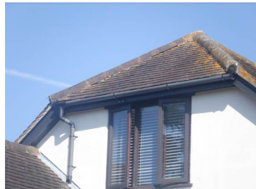
Photograph 6. Gaps in hip tiles on the rear roof
