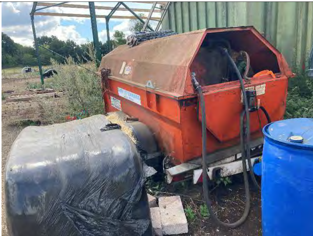
Photograph 18 – Portable fuel bowser situated south of Tank 2 (facing east)
