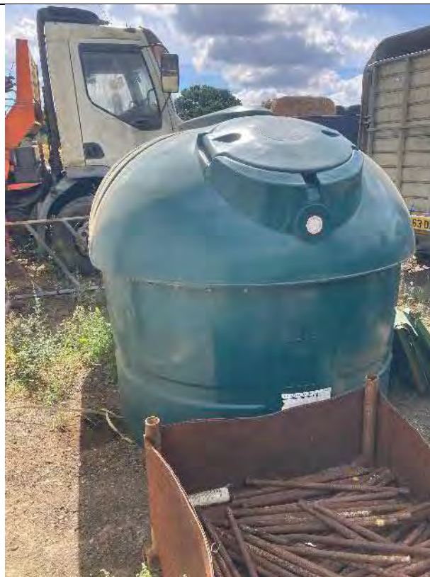
Photograph 16 – Tank 1 (bunded fuel tank) adjacent to Barn 3 (facing south).
