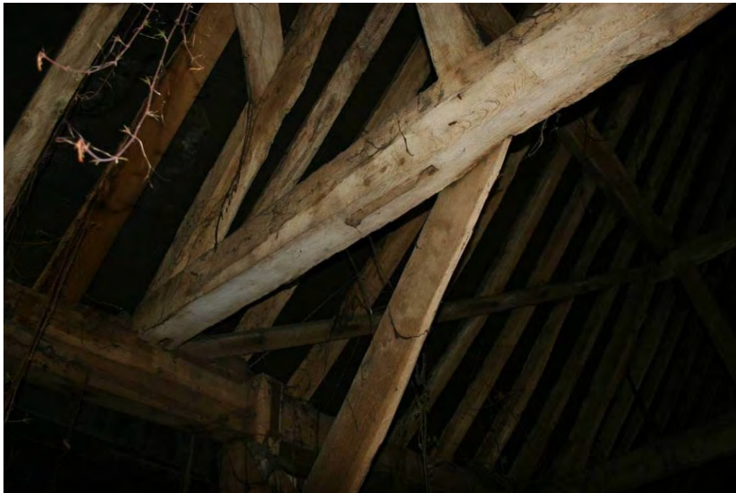
Detail of the displaced storey post and tie-beam assembly.
