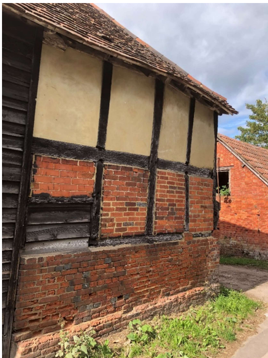
Figure 29: Photo of unit 5 south east corner panels
