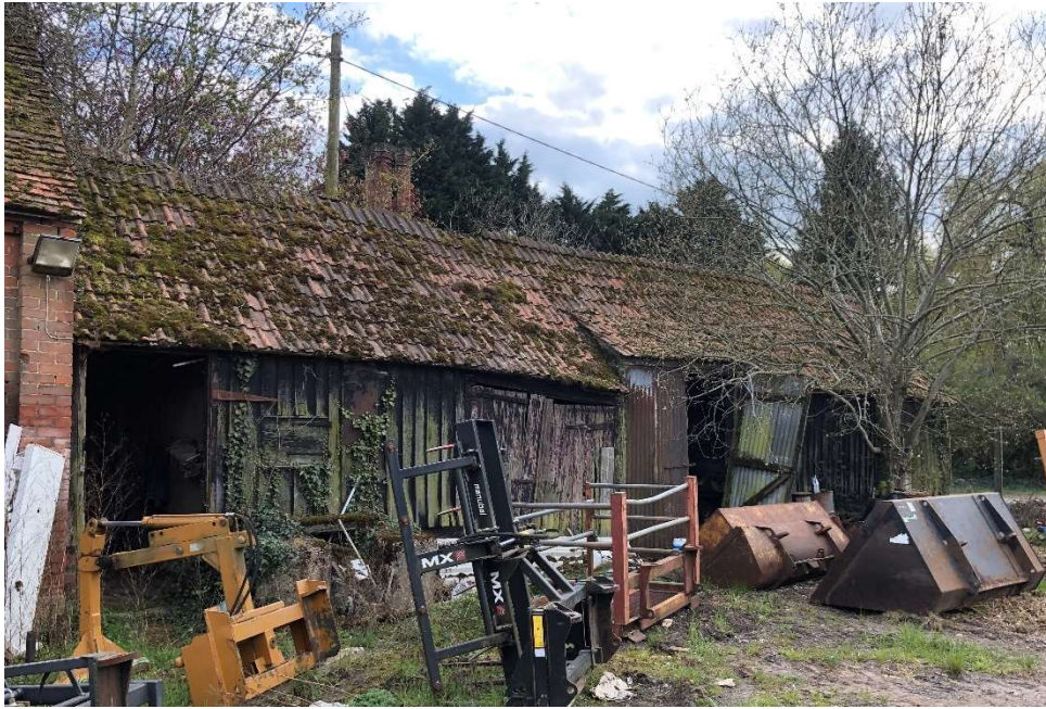
Figure 17: Unit 1 west lower timber section to be replaced
