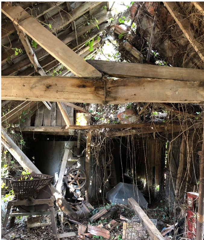
Figure 8: Internal view of Unit 3 showing decay and overgrowth
