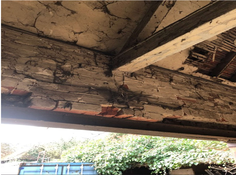
Figure 5: Brickwork collapsing and steel beam over entrance to unit 1
