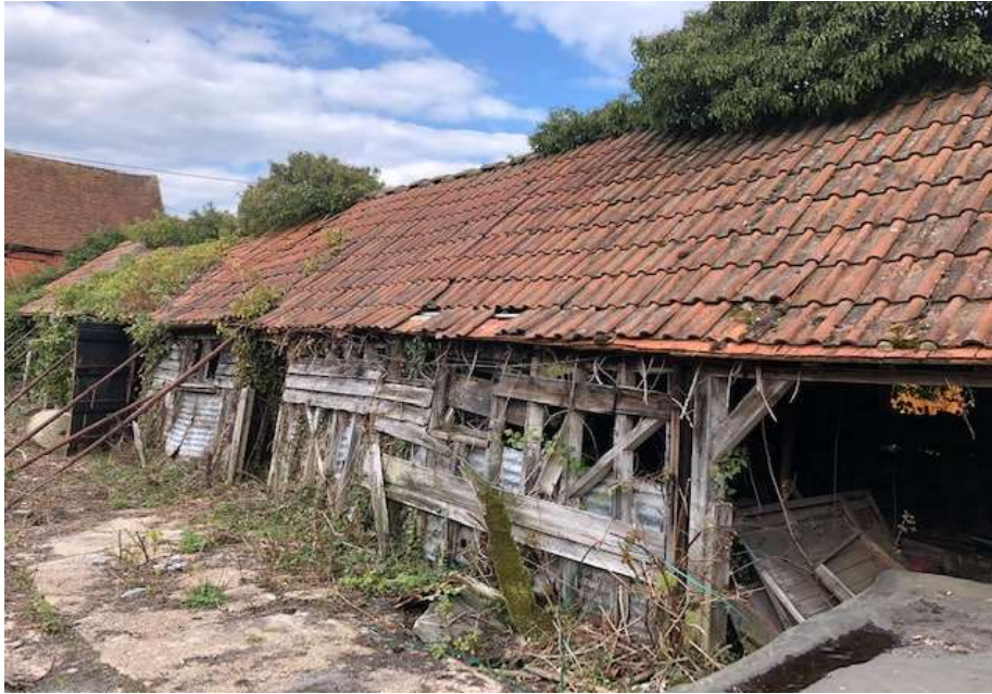
Figure 7: Courtyard view of unit 3 in state of collapse and temporarily propped
