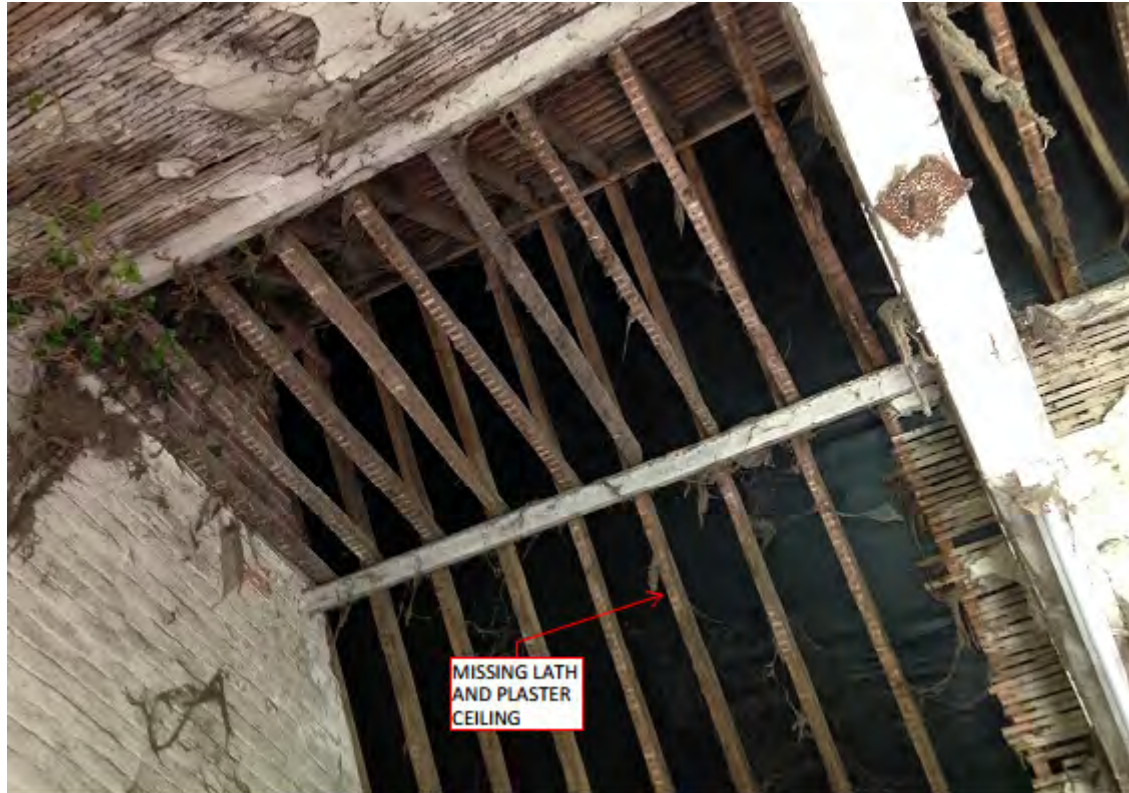
DEFECTS OBSERVED IN BUILDING 'D' & 'E'
