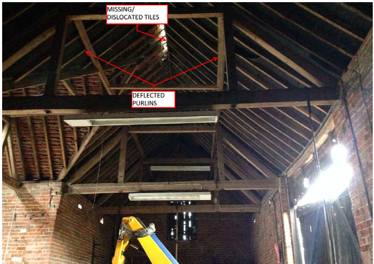
DEFECTS OBSERVED IN BUILDING 'K'
