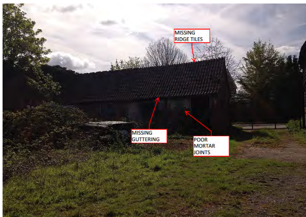
DEFECTS OBSERVED IN BUILDING 'K'
