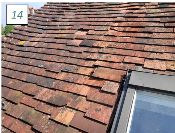
11 – 15: views of the myriad lifted and hanging tiles on the roof
