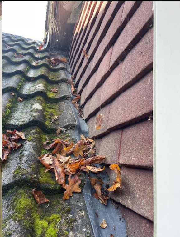
Photograph 22: Gaps between flashing and hanging wall tiles.
