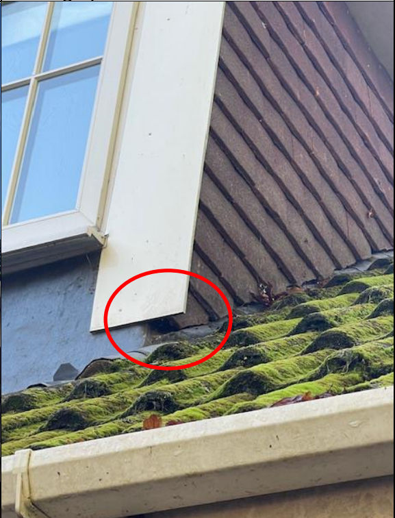
Photograph 4: Gaps at the edge of the dormer.
