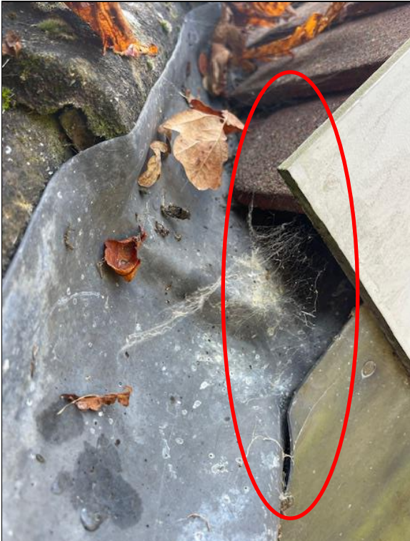
Photograph 21: Gaps between flashing and hanging wall tiles.
