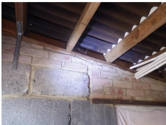
Photograph 3. Timbers sealed to brickwork walls and foam (Outbuilding 1).
