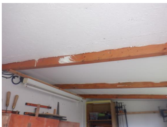
Photograph 9. Plaster boarded walls and ceiling fully sealed (Outbuilding 3).
