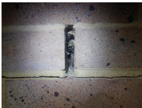
Photograph 14. Features of limited extent within slits filled with debris (Rear elevation of the garage).
