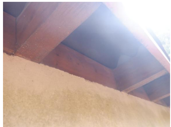
Photograph 2. Gaps within grooves of corrugated sheets blocked by felt (Outbuilding 1).
