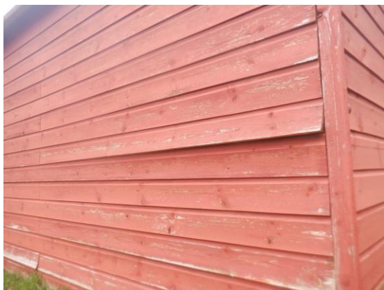
Photograph 6. Gap of limited extent behind lifted timber cladding (Outbuilding 2).
