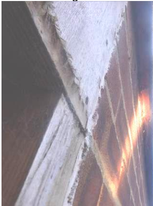
Photograph 7. Superficial gap behind fascia to the rear of the garage.
