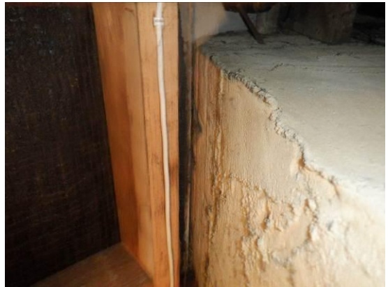
Photograph 12. Daylight in gap between felt and chimney
