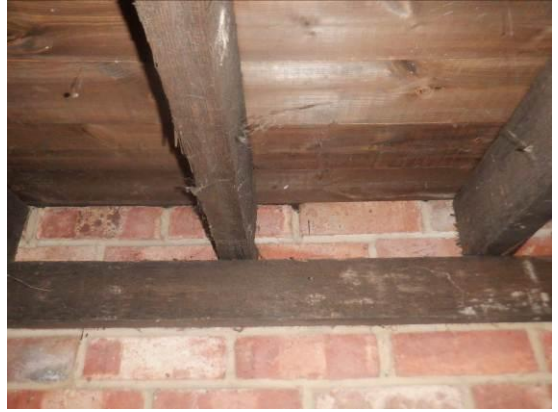
Photograph 18. Gaps between blockwork and roof.
