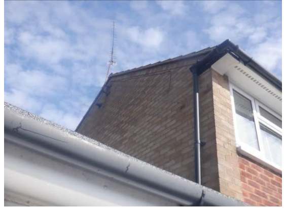
Photograph 6. Tightly fitted uPVC soffits to the front and rear.
