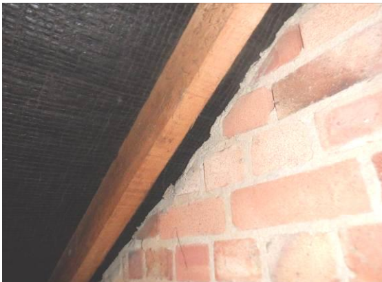
Photograph 15. Gaps around the south east facing party wall.
