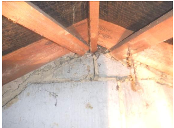
Photograph 16. Gaps around margin in north west facing gable end
