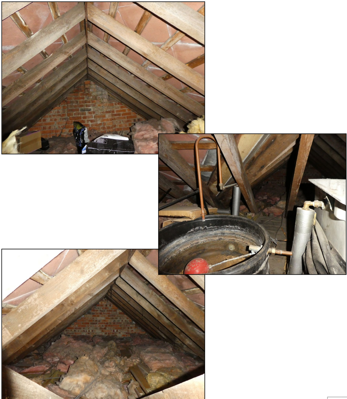
Figure 11. Example of loft space and unlined roof tiles. 37 Hatch Ride, Crowthorne. 27.08.24
