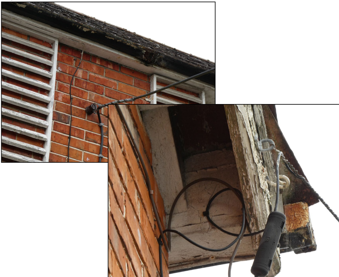
Figure 8. Example of soffits and fascias. 37 Hatch Ride, Crowthorne. 27.08.24
