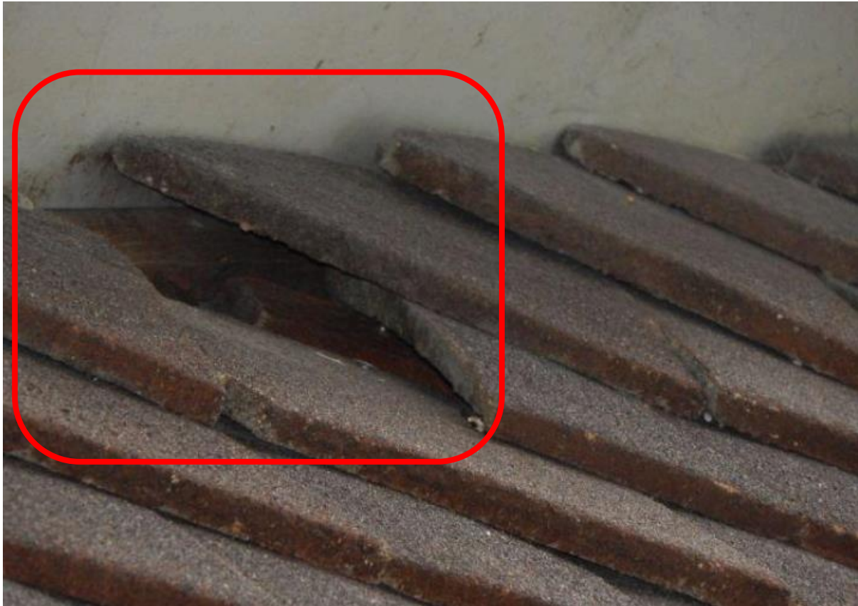
Image 5 – Further missing tiles within the rear South facing elevation which looks to offer further shelter/access opportunities for bats
