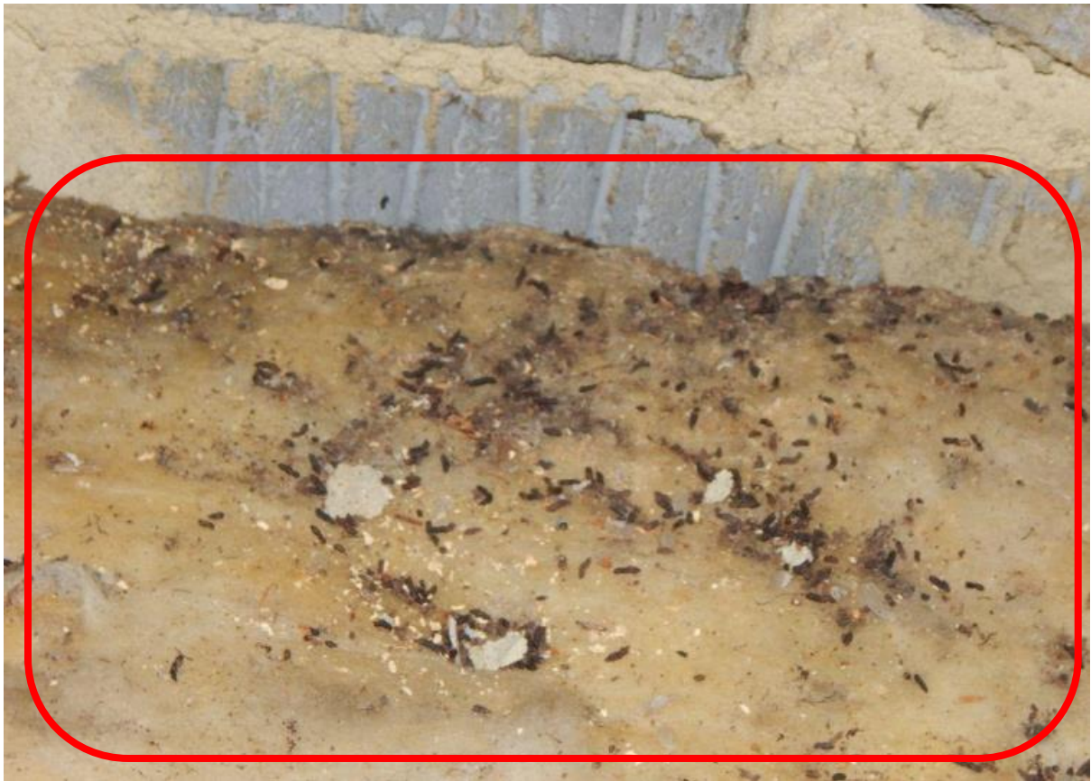
Image 9 – Around 200+ bat droppings observed close to the front and rear gable walls within the upper roof void spaces of the property confirming activity from bats
