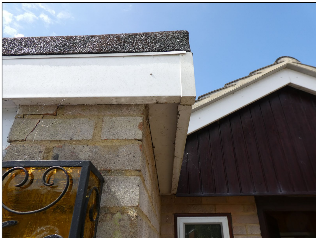
Figure 10. Tightly fitted soffits/fascias on garage. 68 Arthur Road, Wokingham. 12.06.24
