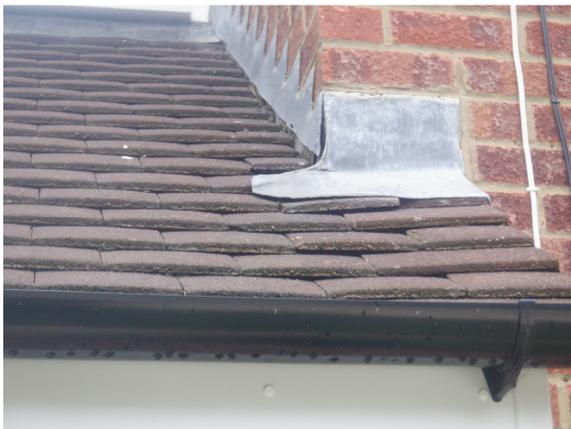
Photograph 7. Partially lifted lead flashing (rear elevation).
