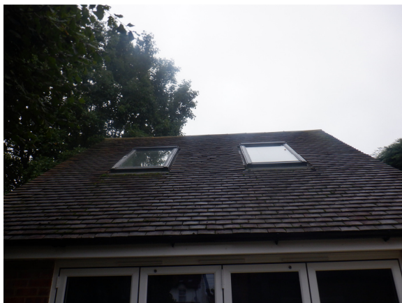
Photograph 11. Raised roof tiles (front elevation of annexe)
