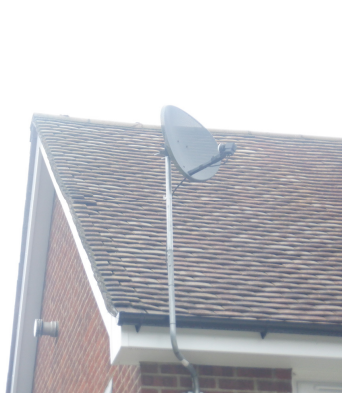
Photograph 3. Raised verge roof tiles along the western verge (rear elevation).
