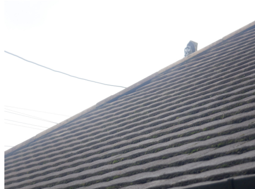
Photograph 6. Crumbling and missing hip mortar (western elevation).
