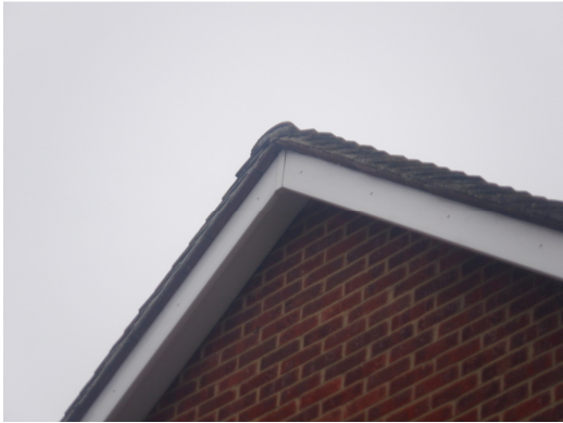
Photograph 5. Superficial crevice within crumbling verge mortar (eastern elevation).
