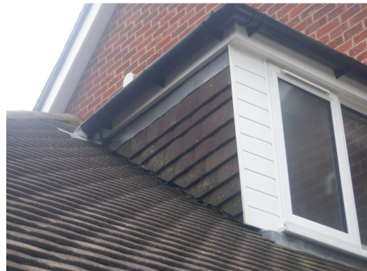
Photograph 8. Tight hanging tiles on dormer window (rear elevation).
