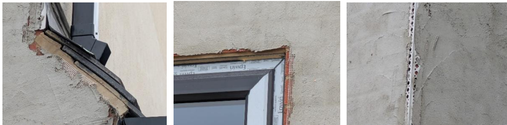
Fig 6: Poor workmanship examples prone to ingress of rainwater
