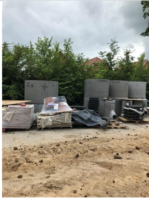
Photo 5. Car park used as storage area
