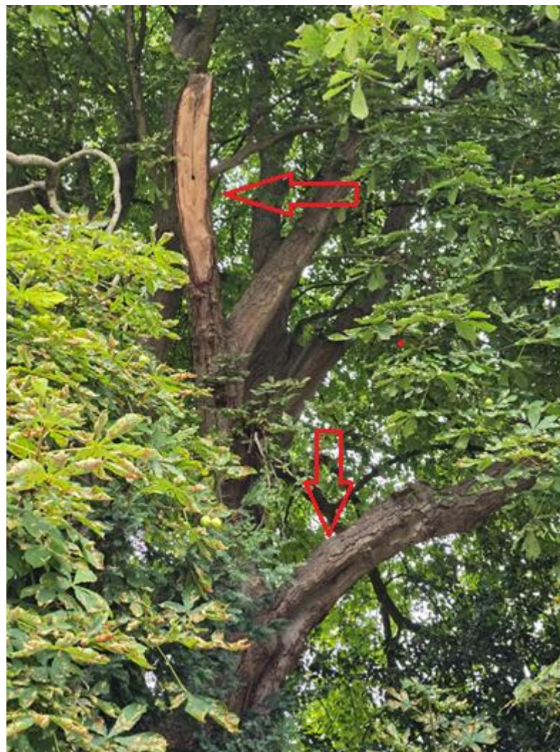
Photo 6 – T2 (Horse Chestnut) broken branch, and raised ridge indicating internal split on lower branch
