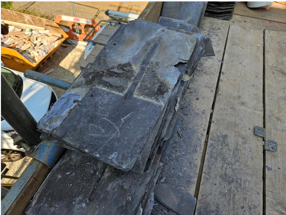
Photo 1: Photo of old slates showing they are not suitable for re-use.
