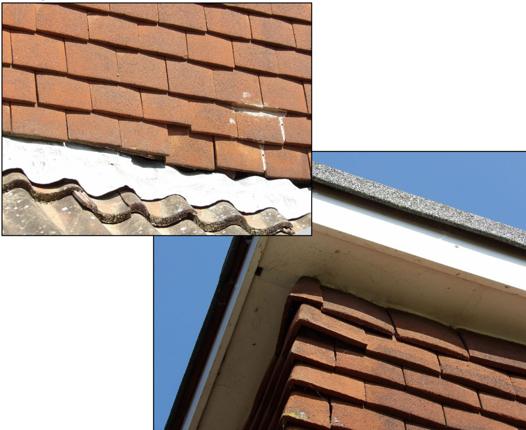
Figure 12. Example moved hanging tiles on rear dormer. 372 Barkham Road, Wokingham. 29.04.25
