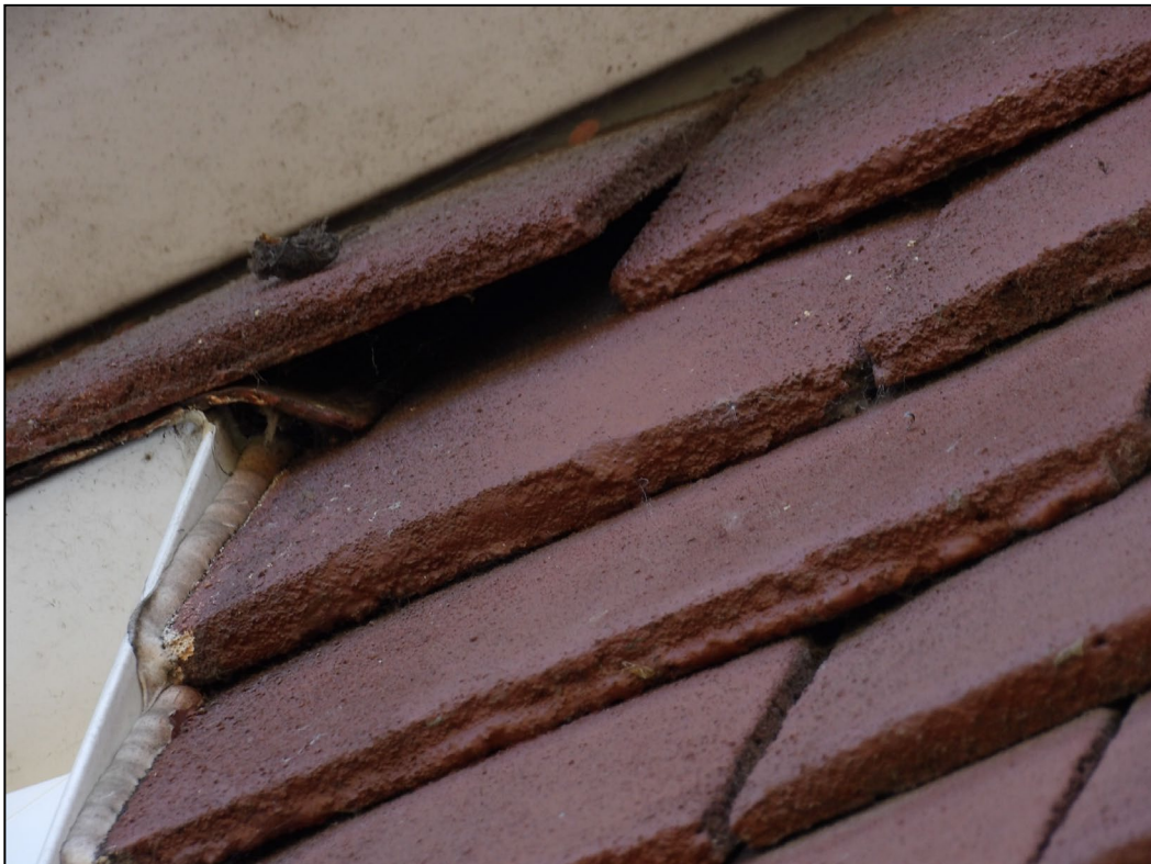
Figure 10. Example gaps hanging tiles on front dormers. 372 Barkham Road, Wokingham. 29.04.25
