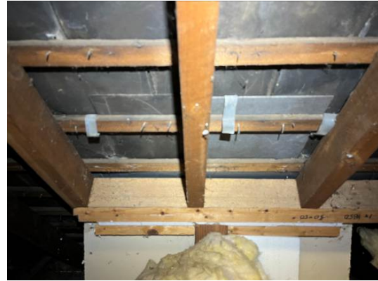
Photograph 12. Unlined roof (Southwest eaves space).
