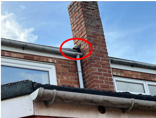
Photograph 6. Lifted bitumen felt at the base of the chimney (rear elevation).
