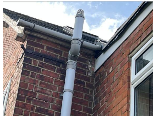
Photograph 4. Hessian-reinforced bitumen felt slightly lifted (southeast elevation).
