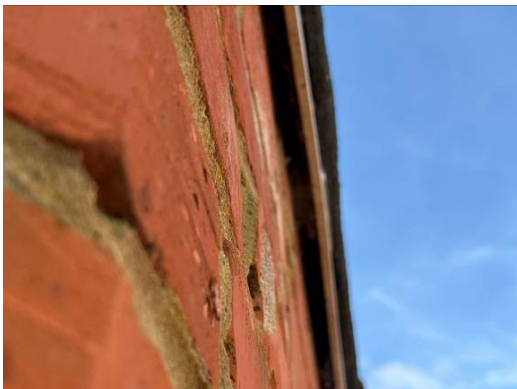
Photograph 10. Gap behind uPVC fascia (rear elevation).
