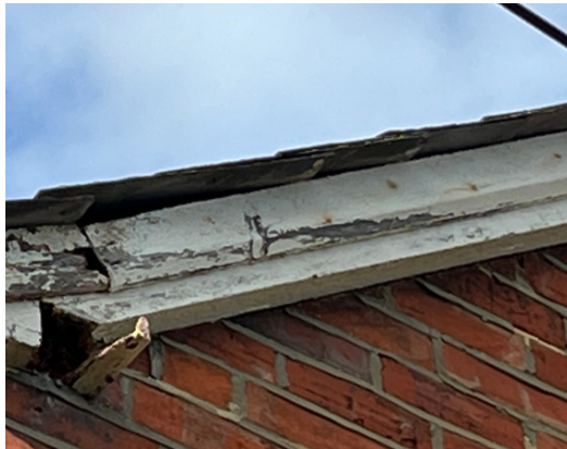
Photograph 9. Gap between timber fascia and verge tiles (southeastern elevation).
