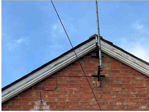
Photograph 7. Gaps between timber fascia and brickwork gable (southeastern elevation).
