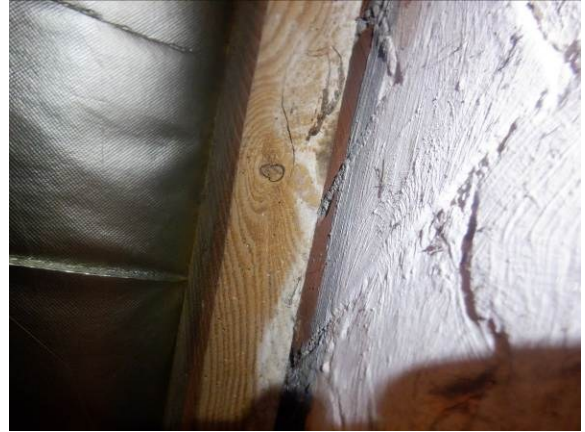
Photograph 13. Gaps between end rafter and brickwork at gable end.
