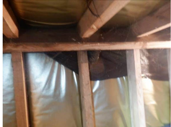
Photograph 9. Heavily cobwebbed ridge and bitumen visible along the ridge in places.
