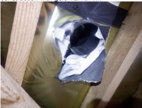
Photograph 10. Gaps around the ventilation pipes in the roof void.
