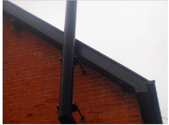
Photograph 6. Verges tightly sealed with a plastic trim.
