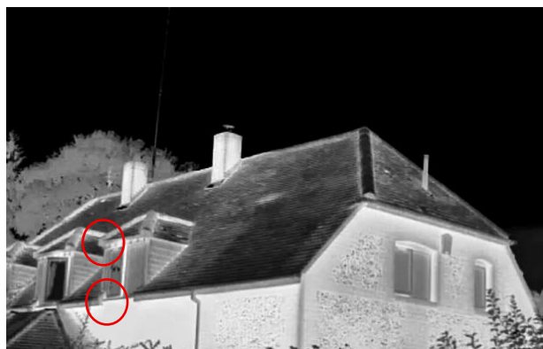
Photograph 3. Soprano pipistrelles emergence points from rear domer (Guide TK61 surveyor location 4).
