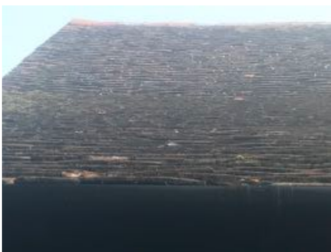
Image 5: Lifted ridge tile on the northwestern aspect
