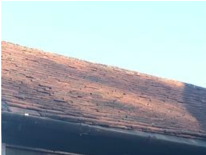
Image 3: A number of lifted roof tiles on the dormer window
