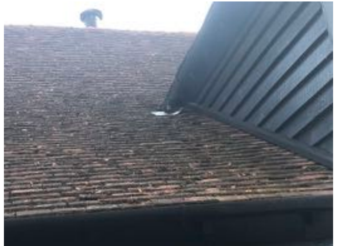
Image 4: Lifted tiles on the northwestern aspect
