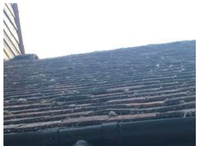
Image 6: Lifted tiles on northeastern aspect with evidence of moss
