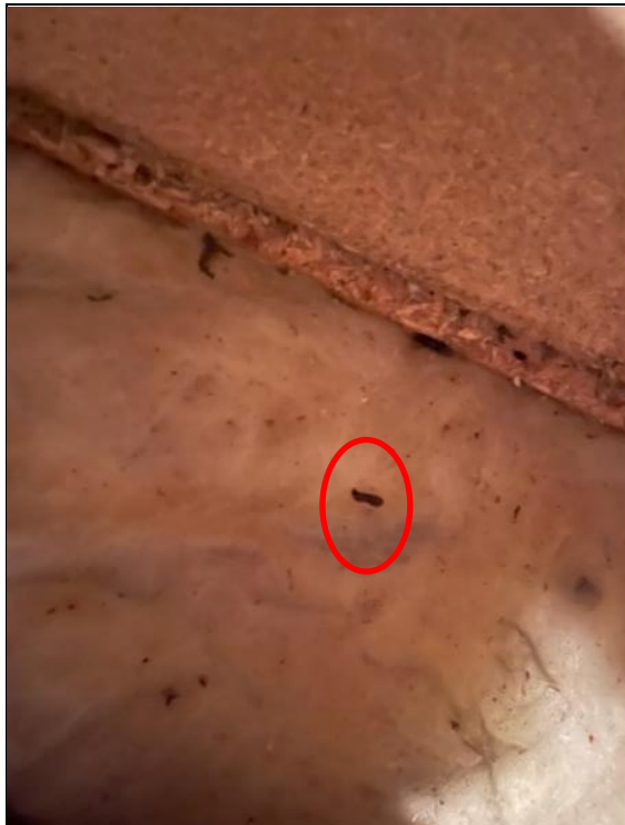
Photograph 17: Bat dropping in loft space.
