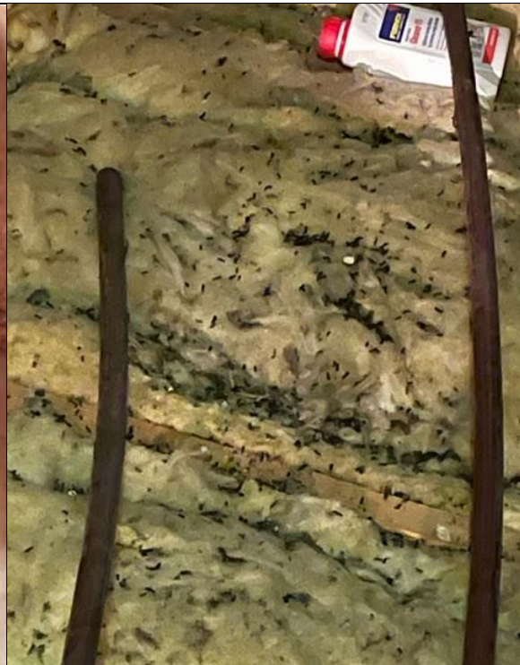
Photograph 18: Large amount of bat droppings in loft space.
