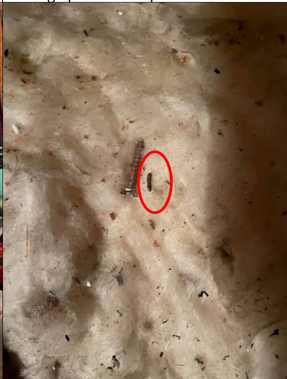
Photograph 12: Bat droppings in main loft space.
