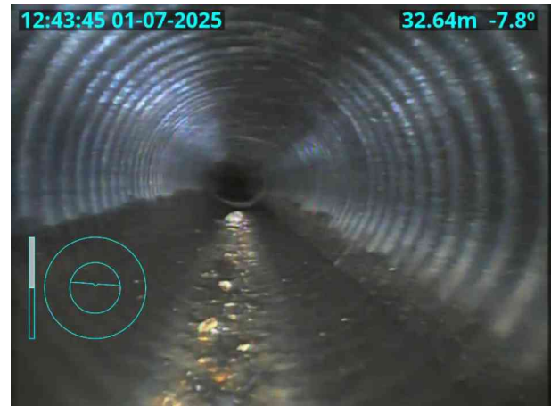
6, 00:03:28, 32.64 m Settled deposits, fine, 5% cross-sectional area loss
