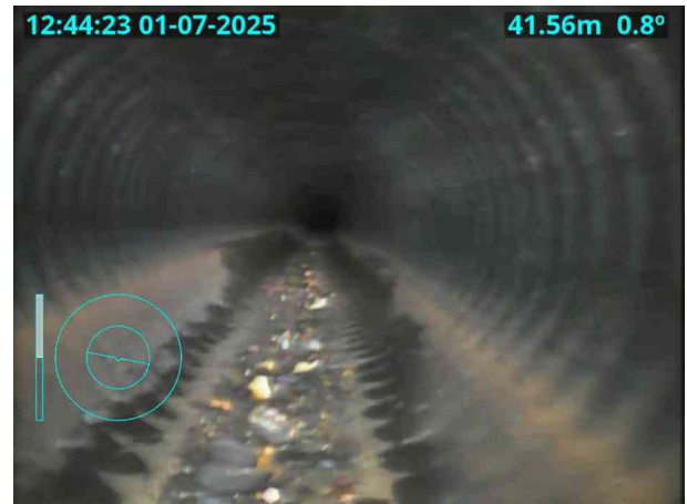
10, 00:04:05, 41.56 m Settled deposits, fine, 5% cross-sectional area loss
