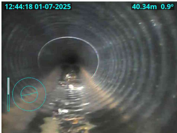
9, 00:04:01, 40.34 m Settled deposits, fine, 5% cross-sectional area loss
