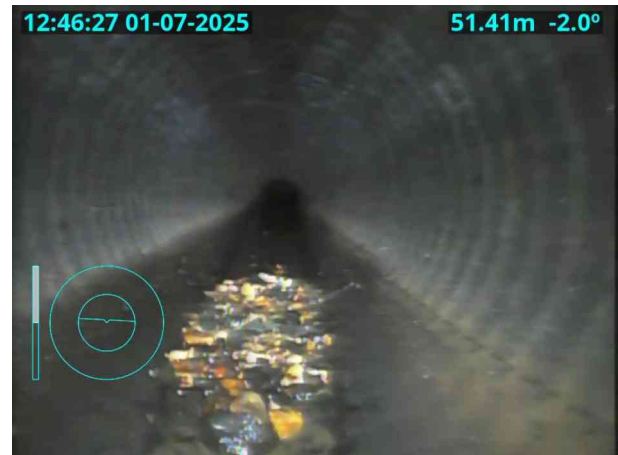
14, 00:06:07, 51.41 m Settled deposits, fine, 10% cross-sectional area loss
