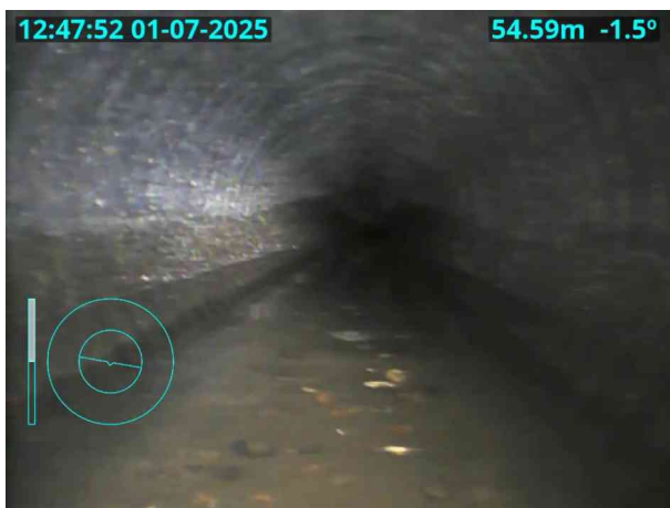
15, 00:07:33, 54.59 m Settled deposits, fine, 10% cross-sectional area loss
