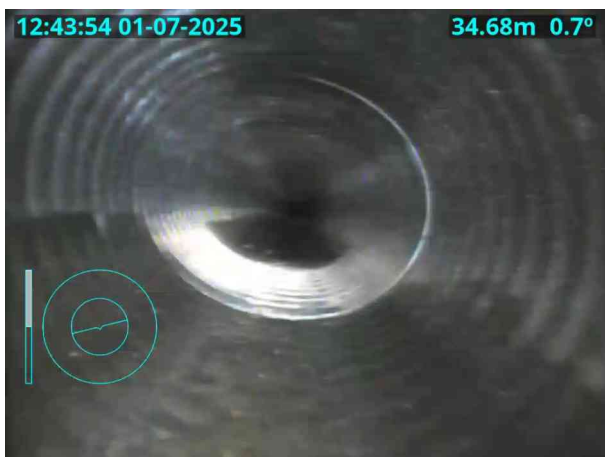
7, 00:03:36, 34.68 m Deformed sewer or drain, 5%
