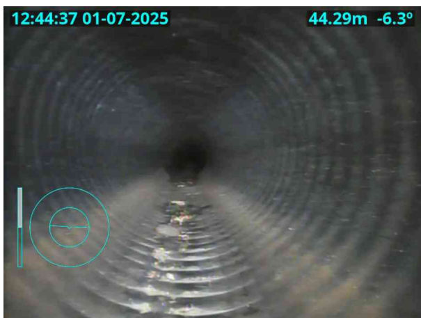
11, 00:04:20, 44.29 m Settled deposits, fine, 5% cross-sectional area loss
