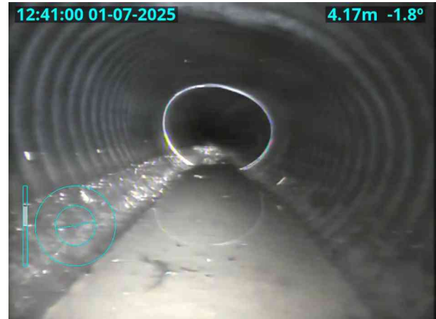
2, 00:00:43, 4.17 m Deformed sewer or drain, 15%
