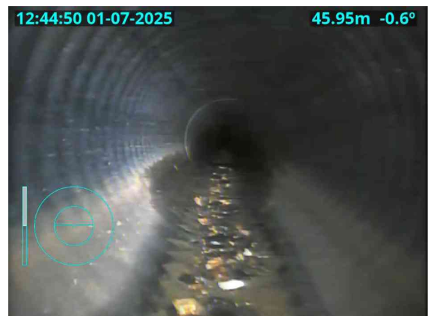
12, 00:04:33, 45.95 m Settled deposits, fine, 5% cross-sectional area loss
