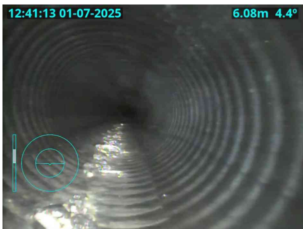
3, 00:00:55, 6.08 m Settled deposits, fine, 5% cross-sectional area loss, start
