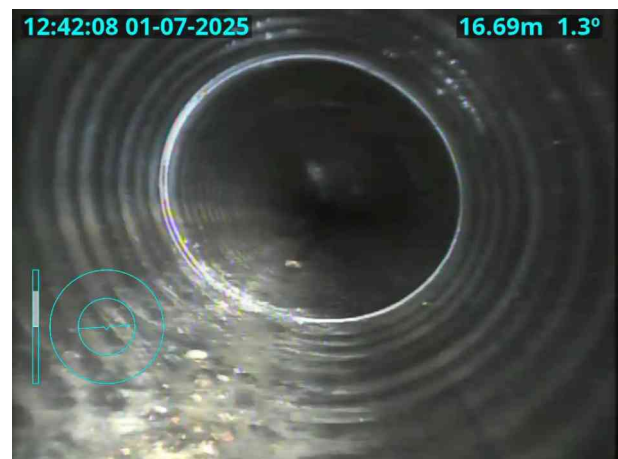
4, 00:01:50, 16.69 m Deformed sewer or drain, 5%
