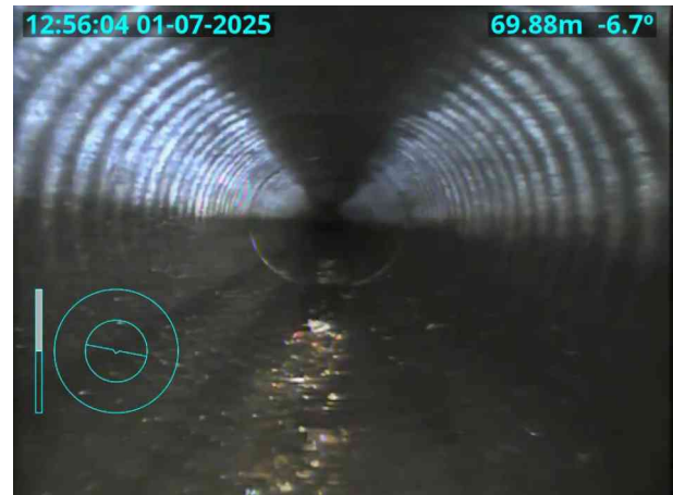
18, 00:13:36, 69.88 m Settled deposits, fine, 5% cross-sectional area loss
