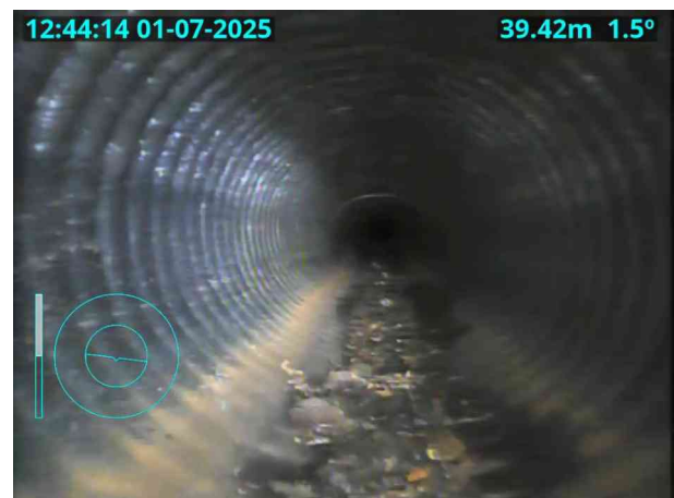
8, 00:03:57, 39.42 m Settled deposits, fine, 5% cross-sectional area loss
