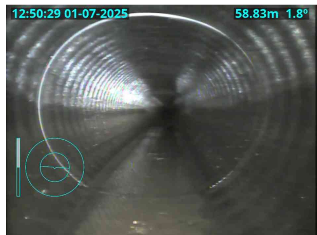
16, 00:09:44, 58.83 m Deformed sewer or drain, 5%
