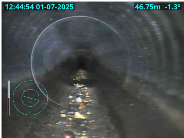
13, 00:04:36, 46.75 m Settled deposits, fine, 5% cross-sectional area loss, start
