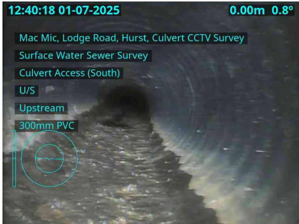
1, 00:00:01, 0.00 m Settled deposits, fine, 10% cross-sectional area loss, start
