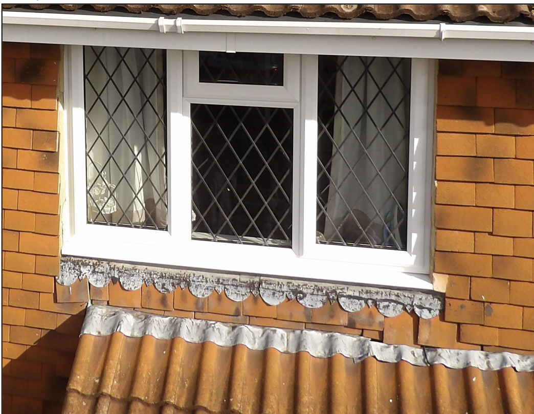
Figure 8. Gaps in hanging tiles below front right window. 8 Barholm Close, Lower Earley. 22.10.24
