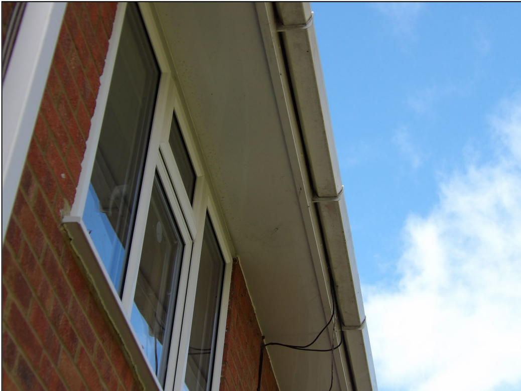
Figure 6. Example of soffits and fascias. 8 Barholm Close, Lower Earley. 22.10.24
