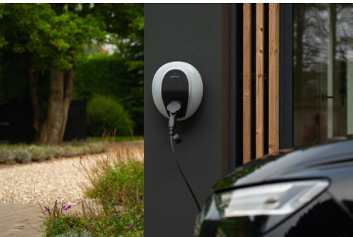
EXTERNAL CAR CHARGING POINT
