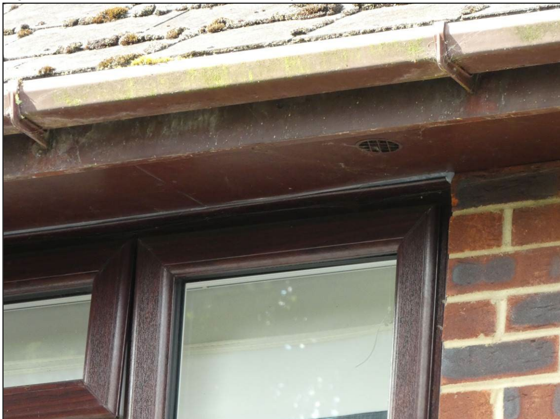
Figure 8. Soffits and fascias. 8 Hunters Way, Spencers Wood, 28.08.24
