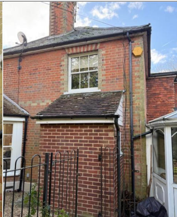
Photograph 10: Lifted roof tiles.
