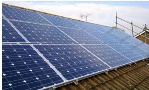
Figure 7 - Roof mounted panels
