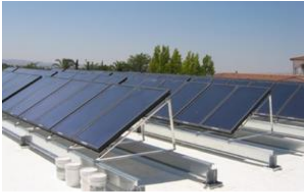
Figure 8 – Frame mounted panels on flat roof
