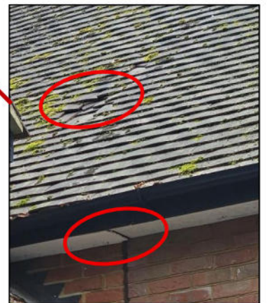
Gaps under roof tiles and around soffits.
