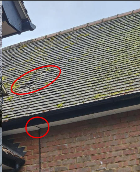
Photograph 6: Gaps under roof tiles and wooden soffits.
