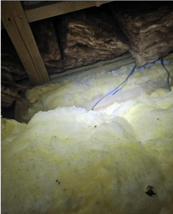
Photograph 9: approximately 50 bat droppings found in the loft space.
