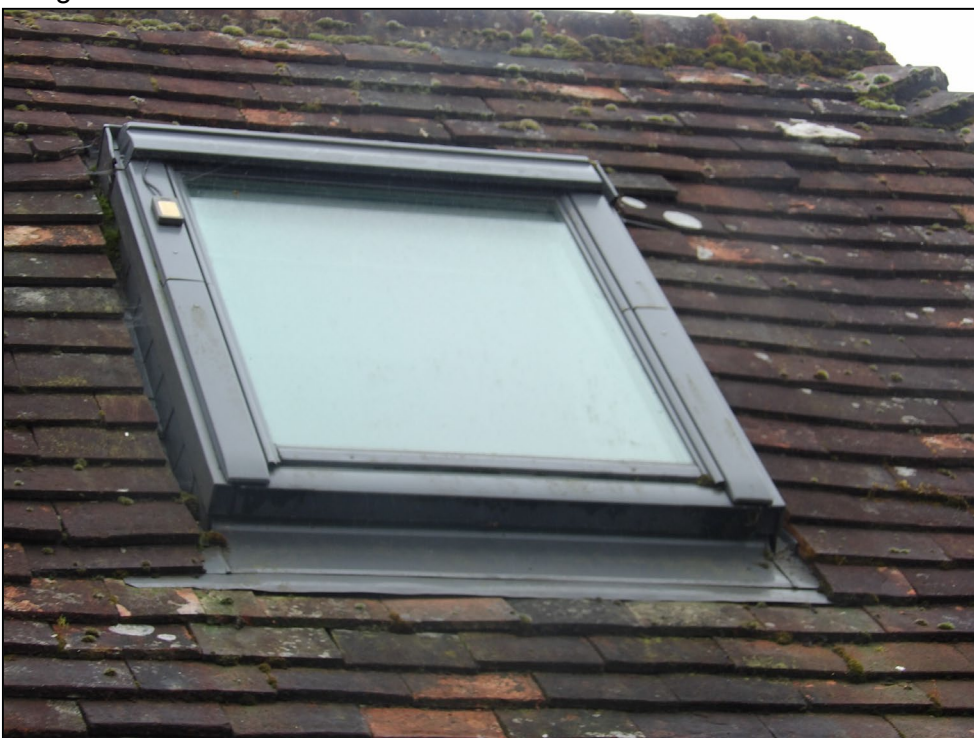
Figure 8. Tightly fitted lead flashing around Velux windows. 195 Victoria Road, Wargrave. 15.04.25
