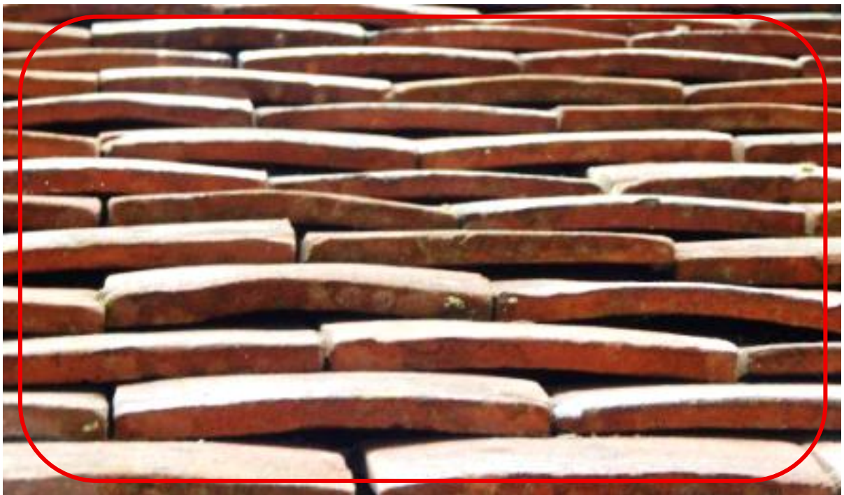
Image 6 – Example of gaps within the rear South facing vertical hanging tiles
