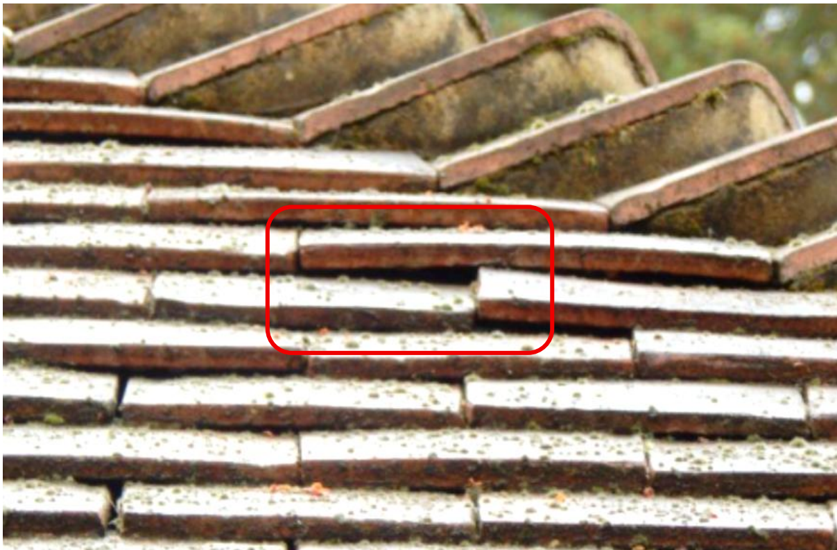
Image 10 – Small number of gaps within the garage roof coverings which look to provide shelter/access opportunities for bats
