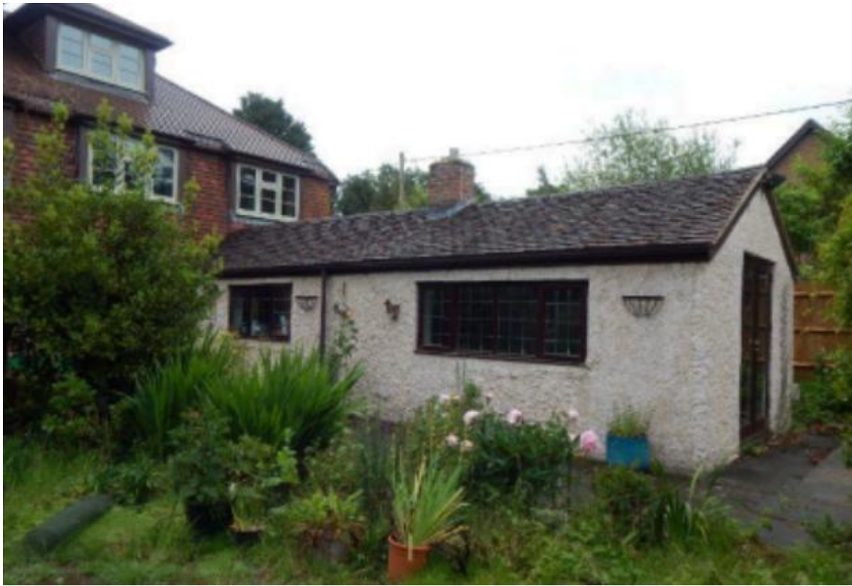
Image 7 – Single storey section to the rear South of the property where further gaps of value across the tiled roof coverings were observed
