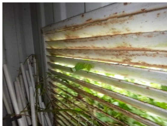
Vented/louvred access (B2).
