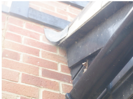
Photograph 7. Heavily cobwebbed gap of limited extent behind lifted lead flashing (front elevation).
