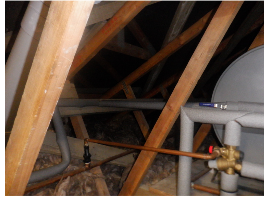
Photograph 11. Southern and western sections of the void inaccessible.
