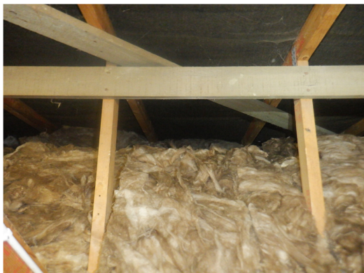
Photograph 13. Eaves blocked and filled by fibreglass insulation.
