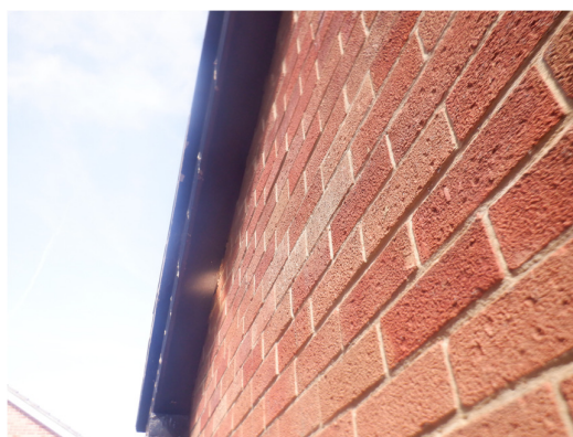
Photograph 9. Gap behind timber soffit (south elevation).
