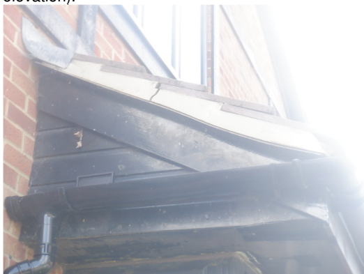
Photograph 5. Superficial crack in verge mortar along the front extension (north elevation).
