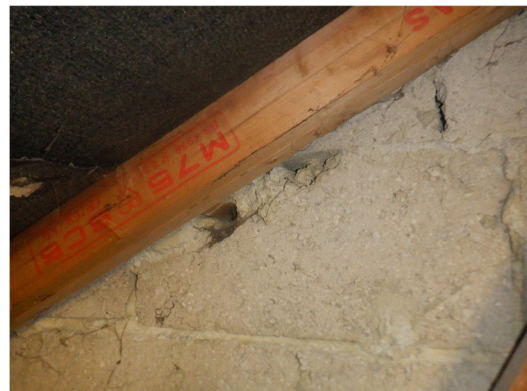
Photograph 14. Slight gaps along the edges of the eastern blockwork gable.
