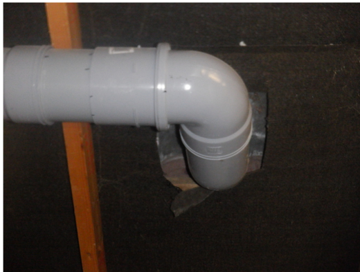
Photograph 12. Tear in felt blocked by a plastic guard.
