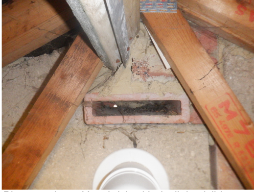
Photograph 15. Vent brick with daylight visible.
