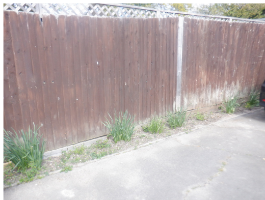
Photograph 6. Gap under timber panel fence along the front driveway.
