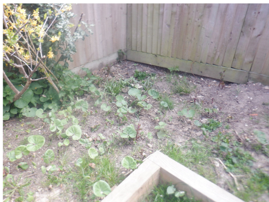
Photograph 5. Gap under timber panel fence in the rear garden.
