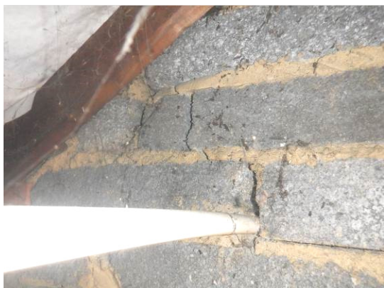
13. Gap around pipe in western gable (roof void).
