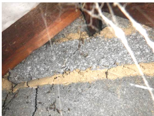
12. Gap at apex of western gable (roof void).
