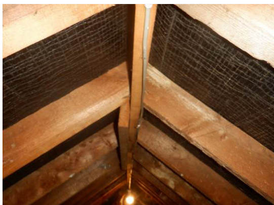
9. Bituminous roof lining and cobwebbed ridge beam (roof void).
