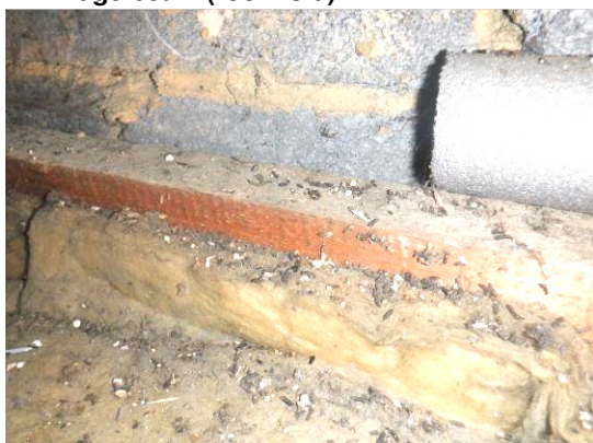
11. Accumulation of approximately 200 small bat droppings at western gable (roof void).
