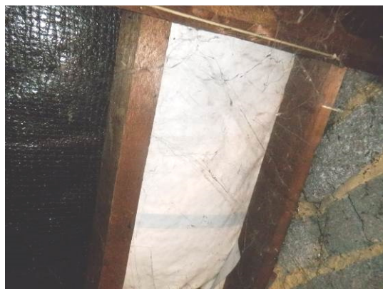
14. Breathable roofing membrane patch (roof void).
