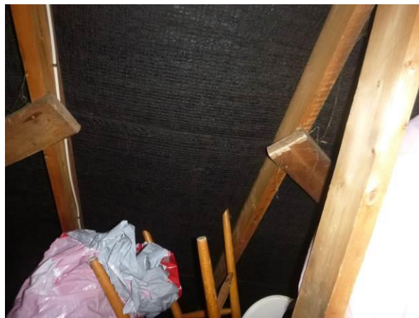
Photograph 12. The intact roofing felt.
