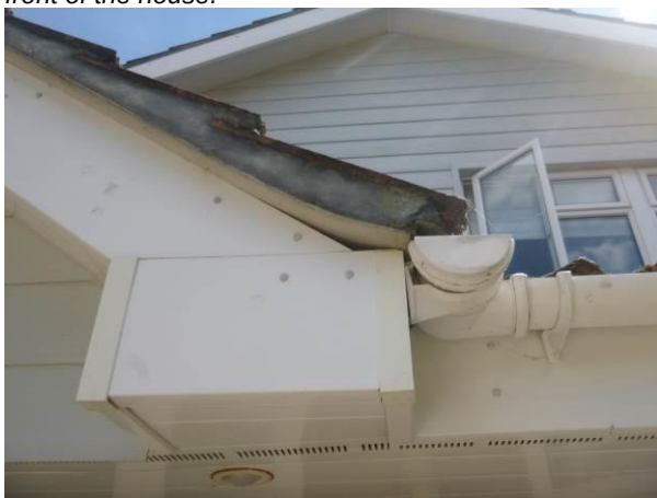
Photograph 9. Cobwebbed gap between the underclocking and soffit box on the front porch.
