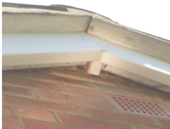
Photograph 8. Heavily cobwebbed gap being the fascias on the rear gable end of the single storey extension.
