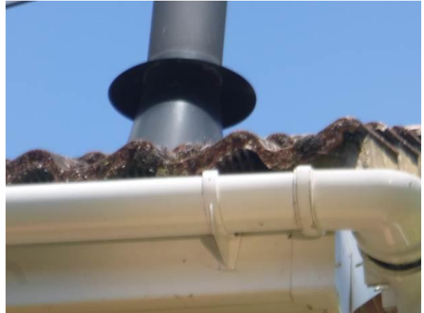
Photograph 4. Mesh present under bottom row of roof tiles.
