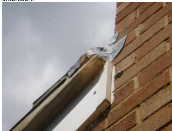
Photograph 10. Cobwebbed gap under the lead flashing at the western side of the house.
