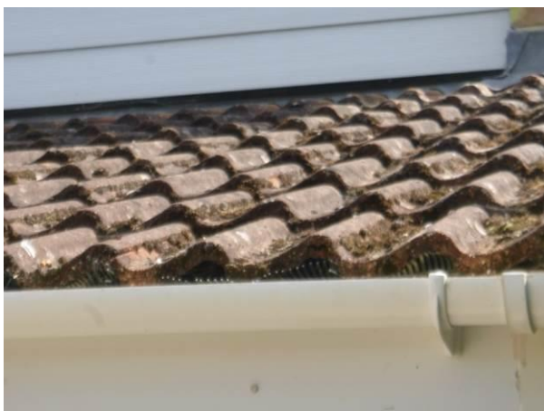
Photograph 7. Mesh present along the base of the roof tiles on the sloped single storey extension to the front of the house.
