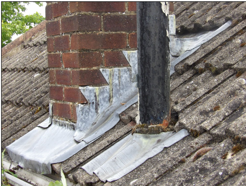
Figure 6. Lead flashing around the chimney and flue. 7 Paddock Heights, Twyford. 27.05.25
