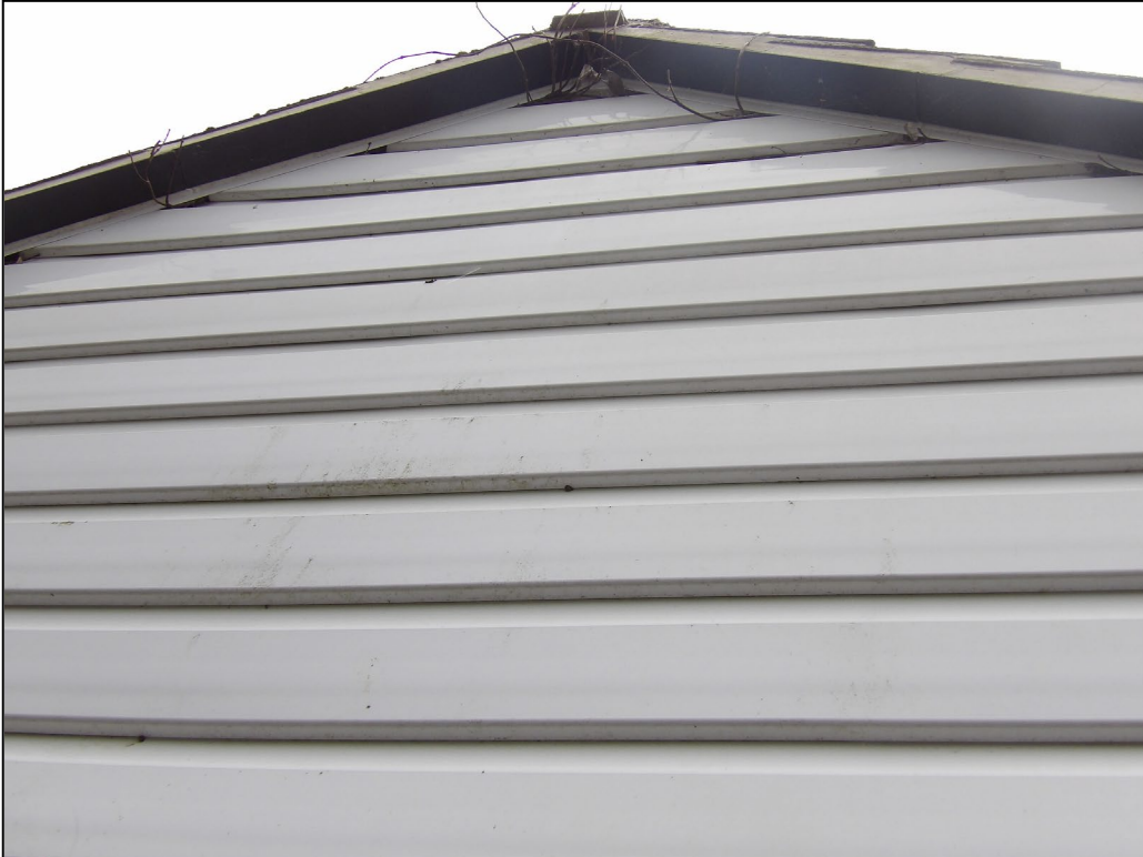
Figure 8. uPVC cladding on rear elevation. 7 Paddock Heights, Twyford. 27.05.25
