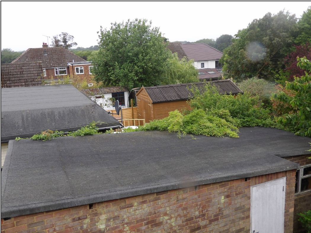
Figure 10. Bitumen covering on garage roof. 7 Paddock Heights, Twyford. 27.05.25
