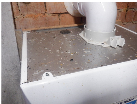
Photograph 1. Additional droppings on top of boiler.
