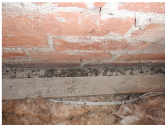
Photograph 1. Additional droppings at eastern gable.
