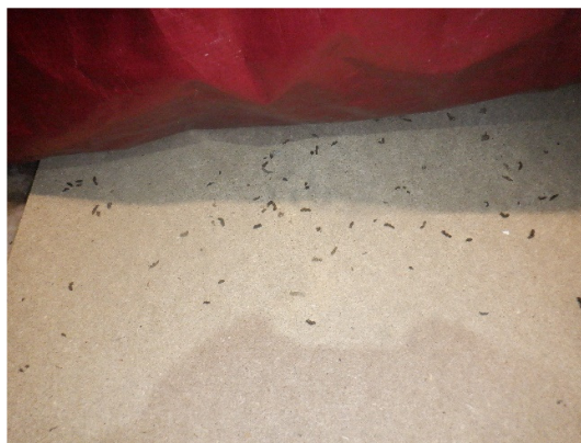
Photograph 2. Additional droppings on boards around stored items.
