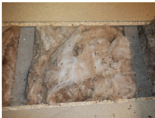
Photograph 2. Additional droppings under ridge beam.
