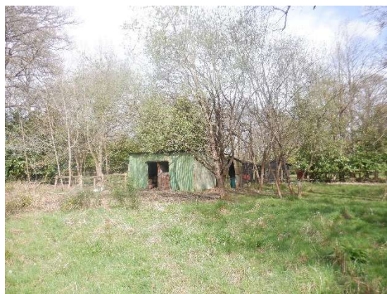
Photograph 4. Dilapidated timber outbuilding (g1d~ 10/12/14/32/203/518).
