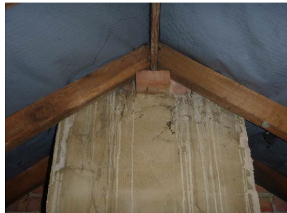
Photograph 11. Cobwebbed rendered chimney at the eastern party wall (roof void).
