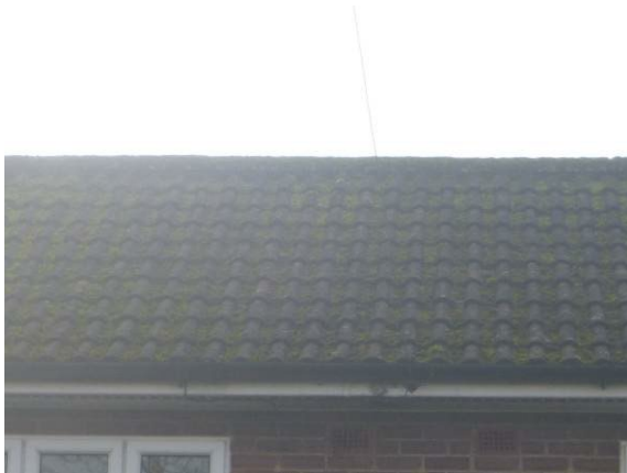
Photograph 3. Mossy roof tiles (front elevation).
