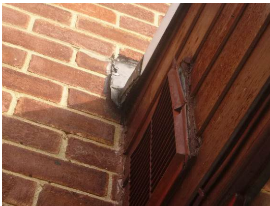
Photograph 7. Slight cobwebbed gap beneath lifted lead flashing on conservatory; negligible roosting potential (rear elevation).
