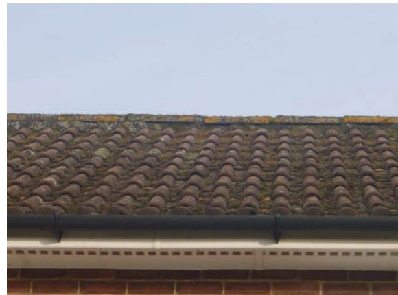
Photograph 4. Crumbling and missing section of mortar below ridge tile (rear elevation).
