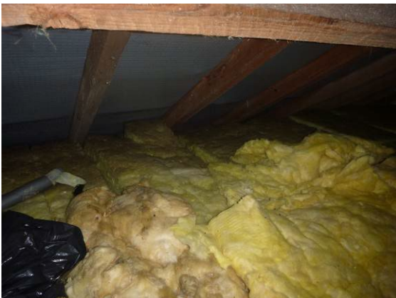
Photograph 10. Fibreglass insulation present up to the eaves, blocking the eaves in places (roof void).
