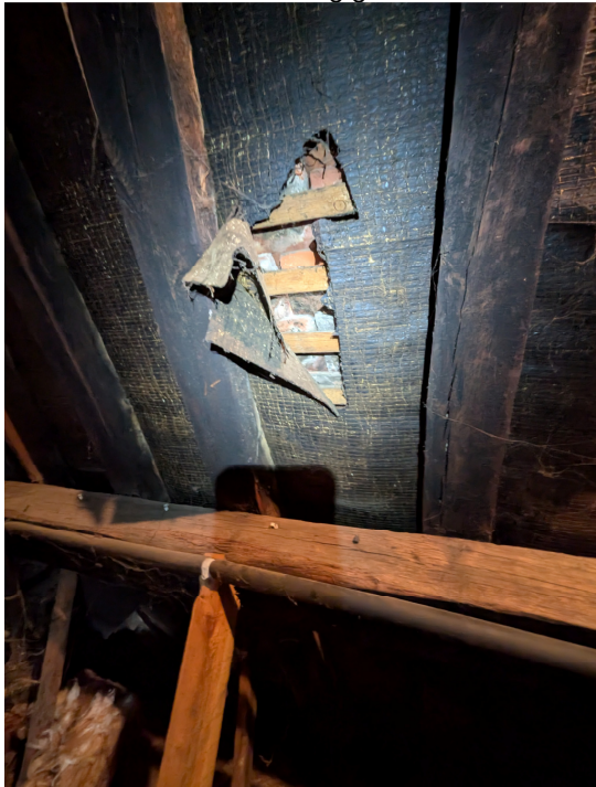
Photograph 5. Tear in the rear roof elevation.
