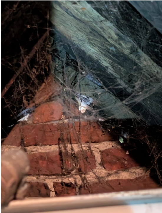
Photograph 3. Daylight visible around the brickwork at the west facing gable end.
