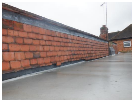
Photograph 11. Gaps behind lifted hanging tiles.
