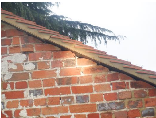
Photograph 10. Gap above brickwork on outbuilding.
