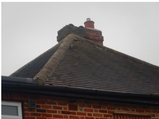
Photograph 6. Lifted roof tiles across main roof.
