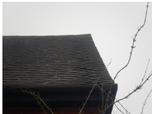
Photograph 7. Lifted verge roof tiles on the northern end of the main roof.
