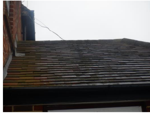
Photograph 13. Gaps under lead flashing on the eastern elevation.
