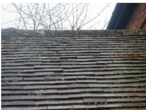
Photograph 8. Multiple lifted tiles on single storey eastern extension.
