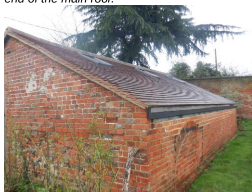
Photograph 9. Multiple lifted tiles on outbuilding.
