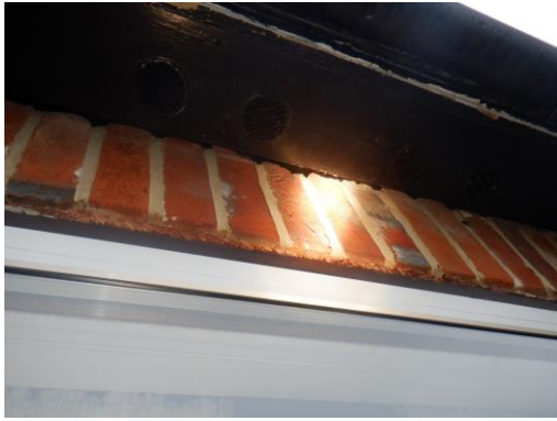
Photograph 12. Gaps behind soffits on the rear elevation of the western extension.
