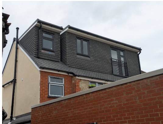
Fig 4: Two Obtrusive Dormers As-Built Note stack pipe
