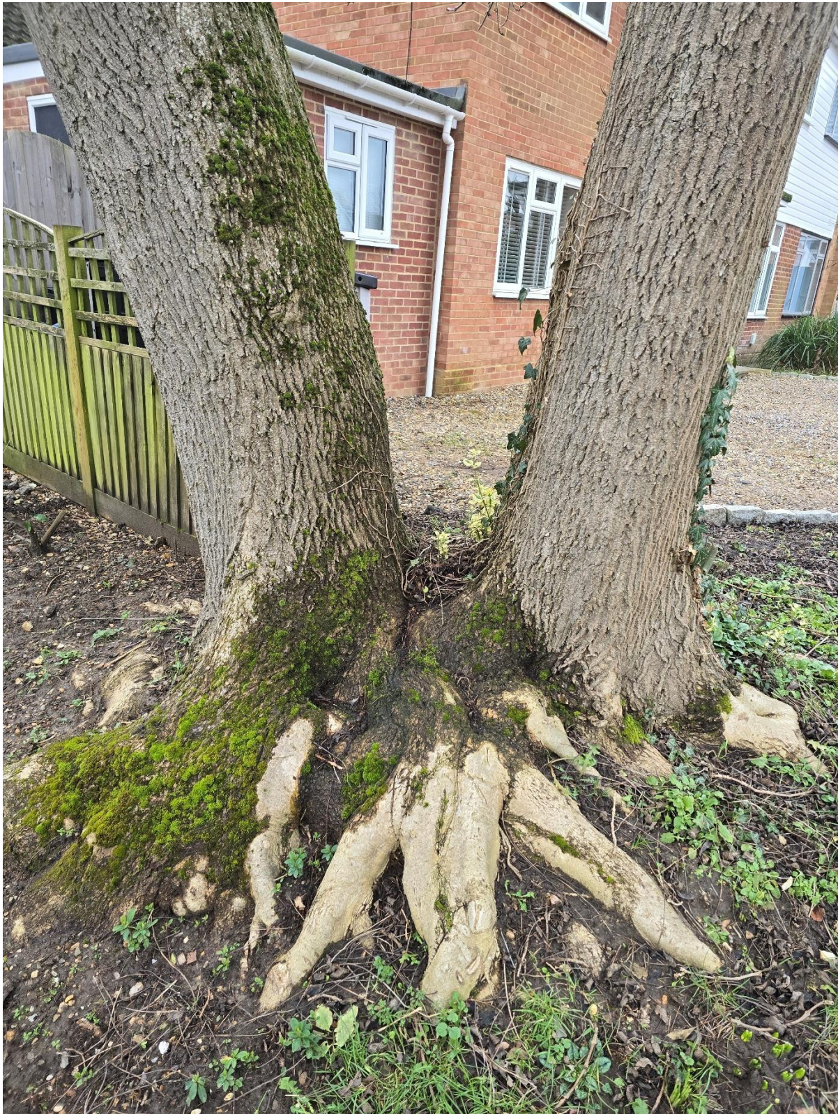
Photo 1 – Exposed surface roots at base
