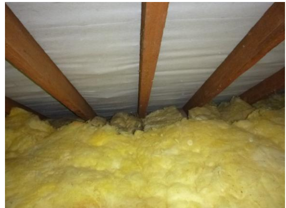
Photograph 13. No fibreglass insulation in eaves.
