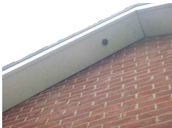
Photograph 10. Narrow gaps behind uPVC soffits on northern gables (rear elevation).
