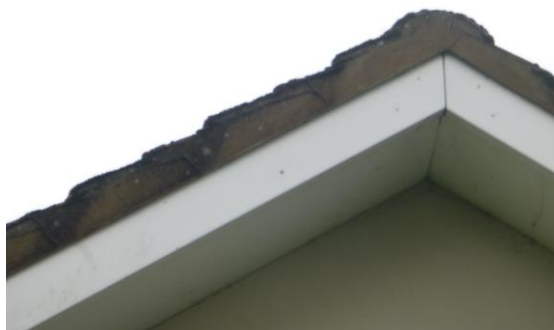
Photograph 5. Fully intact verge mortar (rear elevation).
