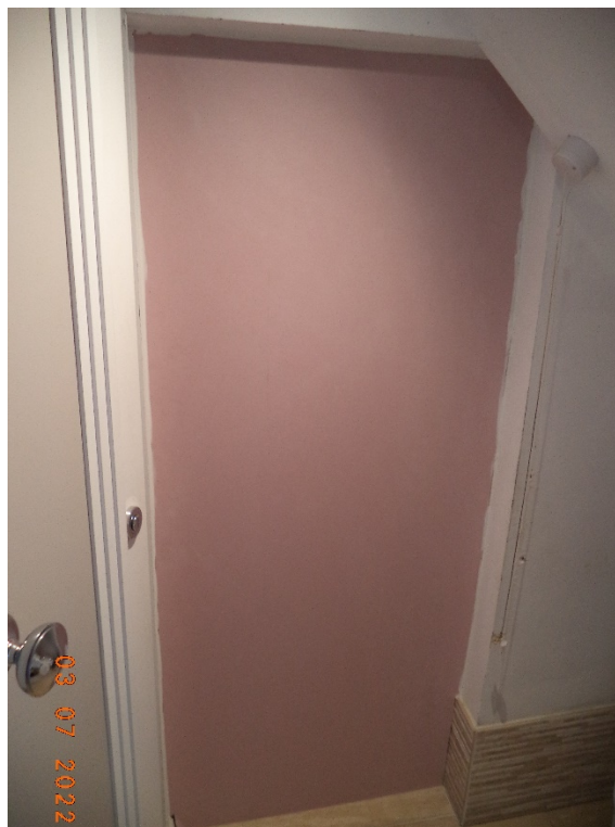
Figure 3: Internal door sealed up, provided by the applicant and dated 03/07/2022
