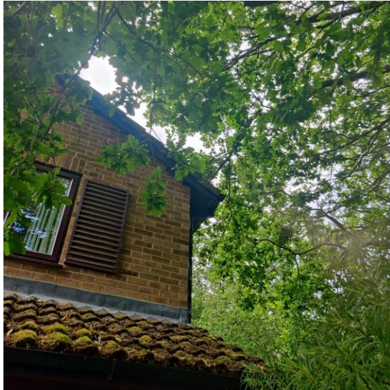
Showing moss build up close proximity to the windows.
